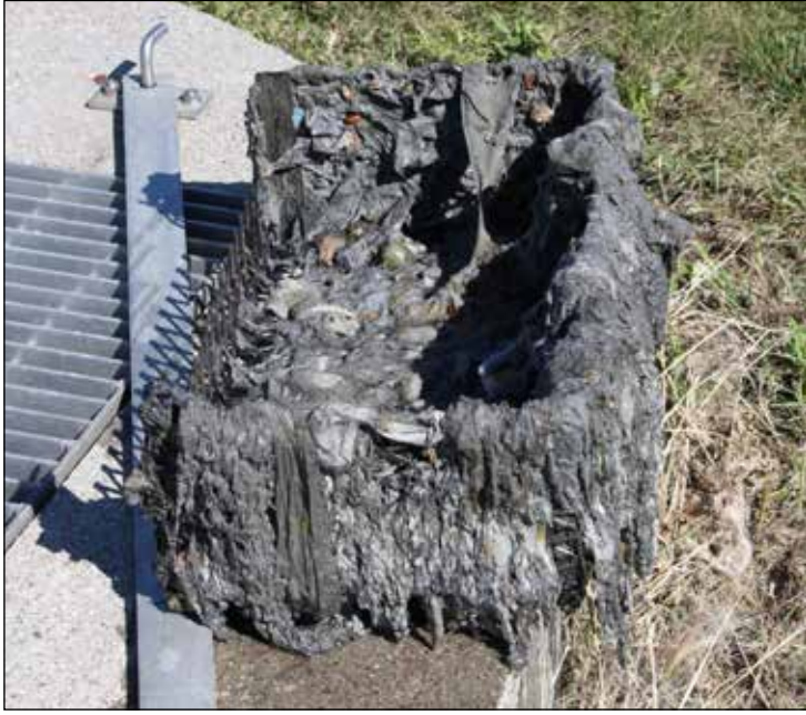
Closeup of dirty screen pulled out from the sewer.
