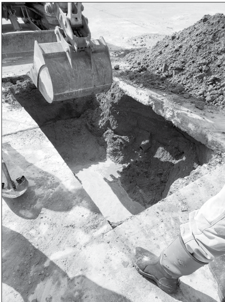
The City of Oklee had to dig up once again the sidewalk on the north side of TJ's Tavern due to a water leak.
