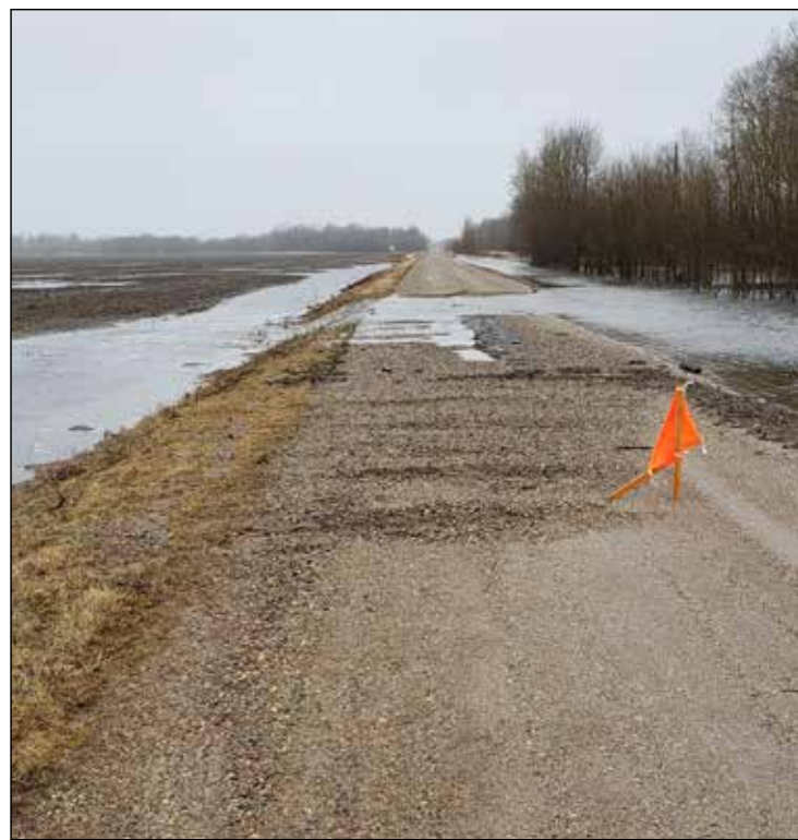
Between Brooks and Erskine on Sunday night, about 4 miles south of Brooks, the water was still running across the road from the rains on Friday night.
