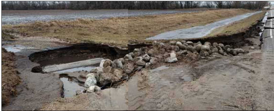
This culvert is along side the damage on Highway 92.
