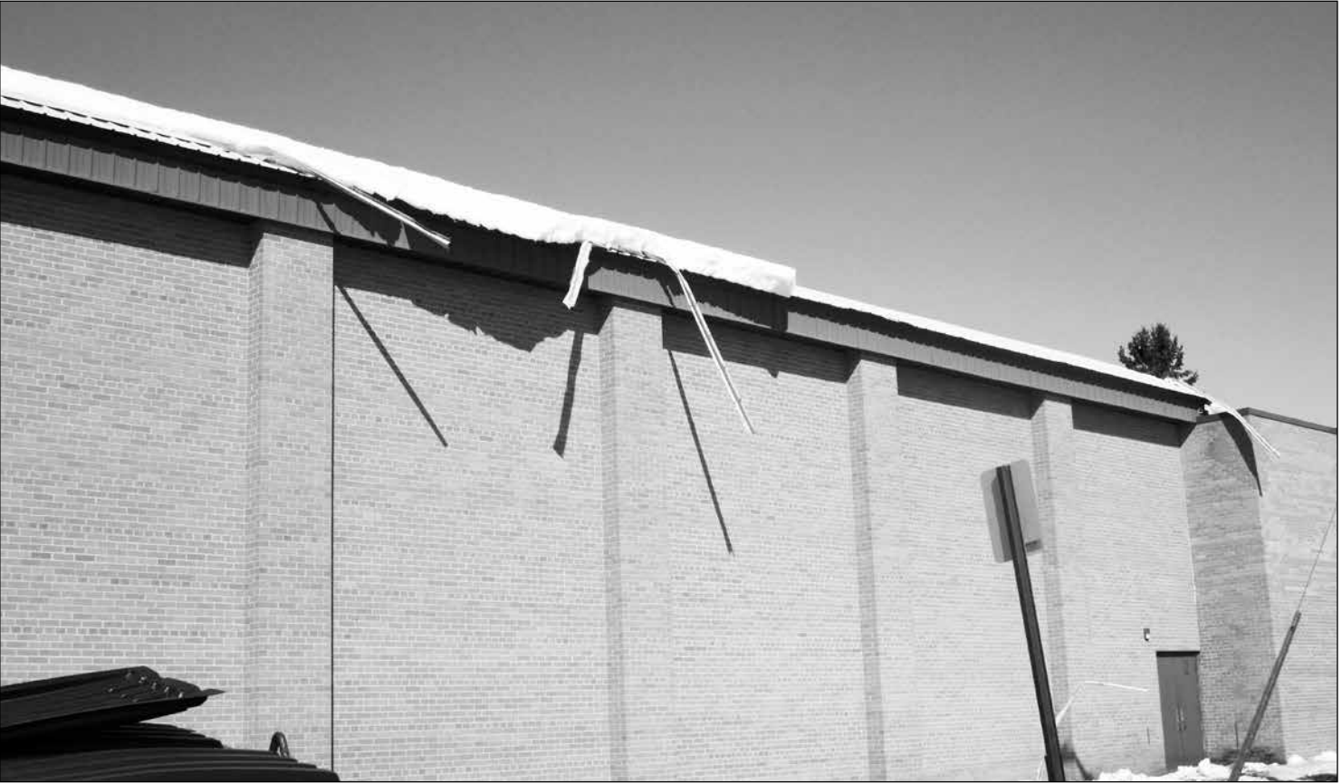
RLCC High School experience some damage to their roof. The snow tore off the snow guards off the roof.
