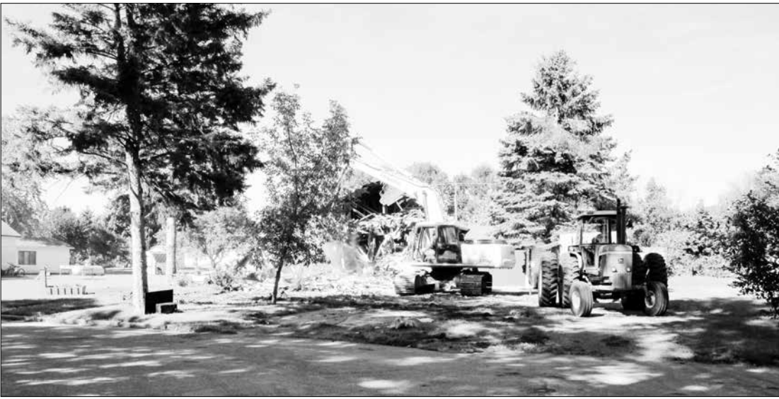
Sadly, the home of Joyce Tougas was damaged beyond repair after a kitchen fire spread soot throughout the home. On August 4th, the house was demolished and Oklee now has one more open lot without a home.
