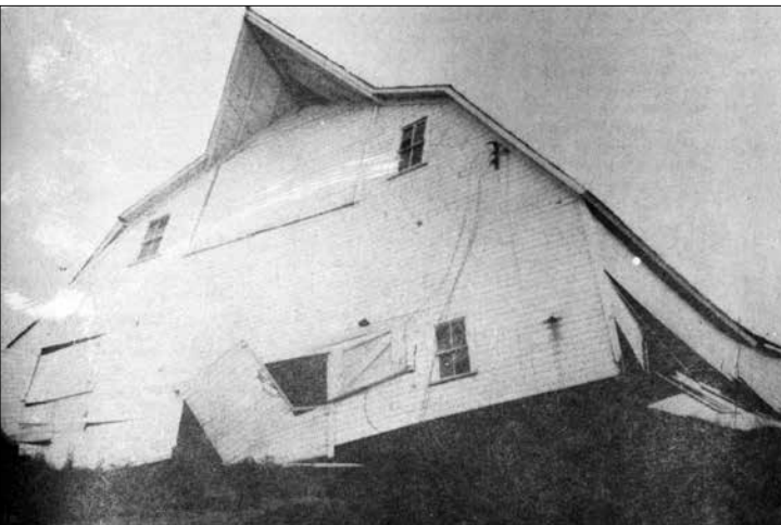
50 years ago...1966: McIntosh area had a brief, but severe storm as newly put up hay filled the hay mow of this barn on the Mrs. Ardella Ostenna farm located almost straight south of McIntosh. A garage close by was also badly damaged.
