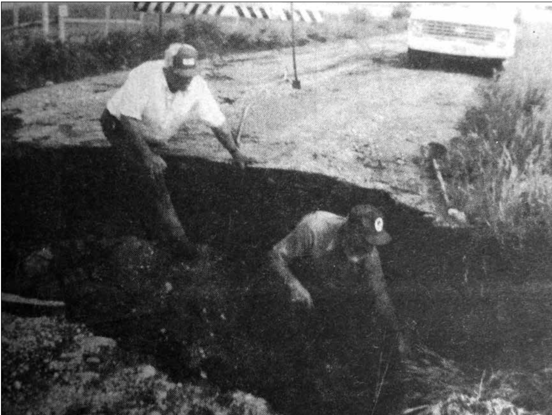
40 years ago...1983: Henry Bartz looks on as his brother, Clifford, who is the King Township road superintendent, examines the damage at the bottom of the collapsed roadway. It took 33 yards of gravel to fill the hole.
