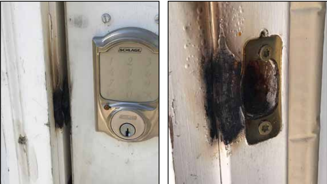
The door locks at Our Savior's Lutheran Church in McIntosh were recently burned in an attempt to gain access to the church located on State Street.
