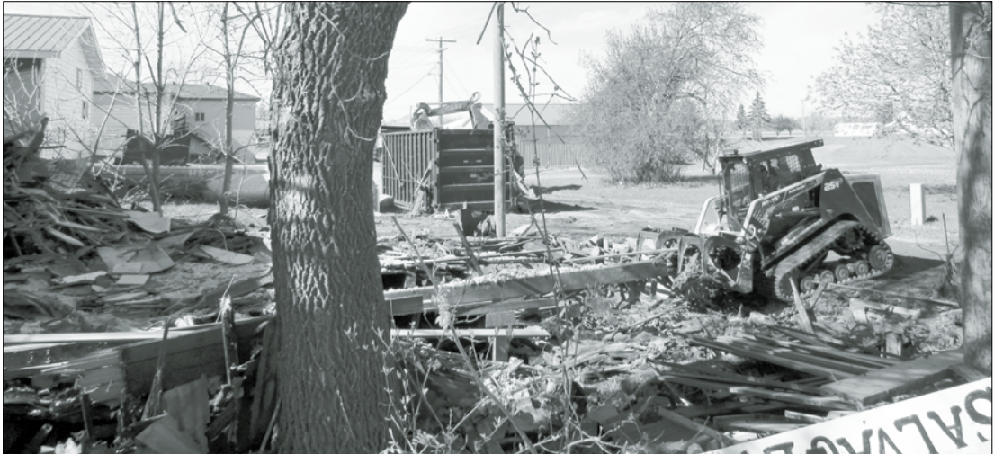
Hedlund Backhoe removed the debris from the fallen building behind the storefront recently purchased by Bryce and Andrea Stordahl in McIntosh.
