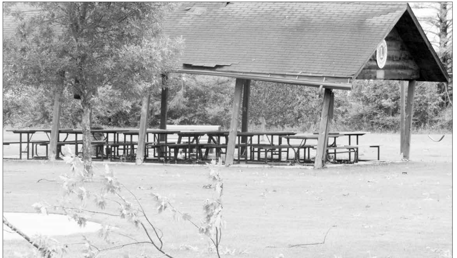
The Winger Lion's picnic shelter was badly damaged as strong storms, and a possible tornado tore through the town of Winger late last Sunday night.
