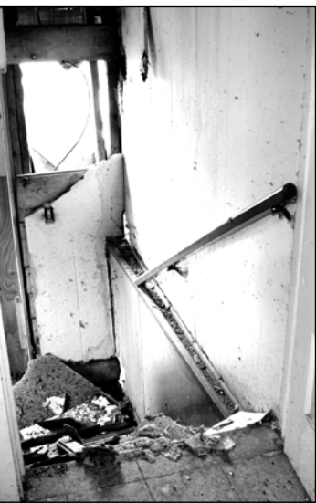
Pieces from the hole in the wall covered the steps.
