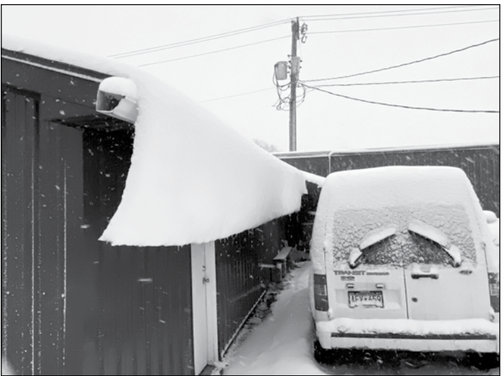
Snow was slowly sliding off the roof. Look out below.
