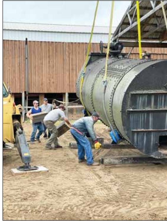
New boiler for the LIRPF.
