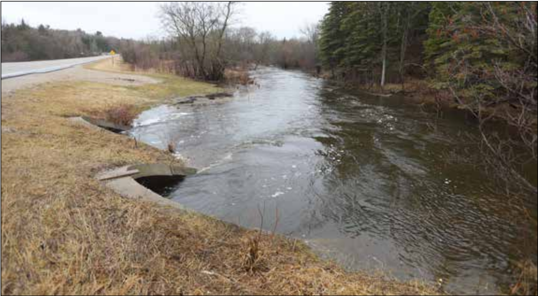
Concrete culverts in Aure with the Clearwater River going through. They held up much better than all the other culverts in the county made of metal.
