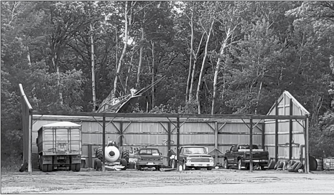
O'Neill's machine shop roof lifted from the building and was deposited in the trees behind the building.
