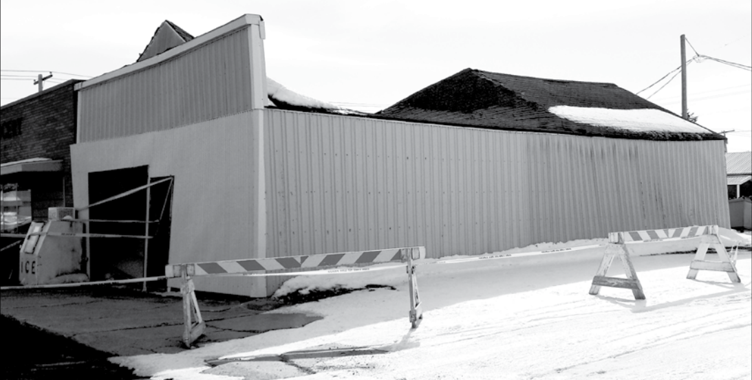
Snow on roofs has caused much damage in the area. In the past couple of weeks, there have been a few buildings that have had their roofs collapse into the building. D & R Grocery owners in Oklee shown above said their building to the north has collapse last Wednesday due to snow. Snow fall this year according to Einar Kvasager's Weather report is now at 69.875 inches for this year. The snow came early this year and there have been very few days where thawing has occurred.
