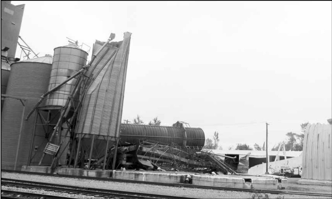
Severe damage to the CHS Elevator in Winger on Monday morning after a severe storm went through town with devastating effects.
