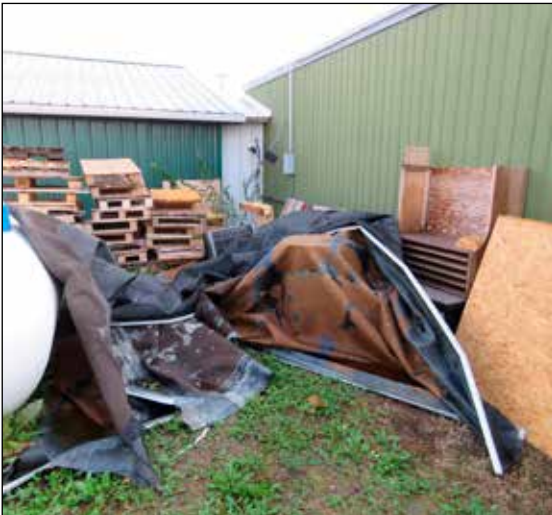
Roof off of Richards Publishing in Gonvick.
