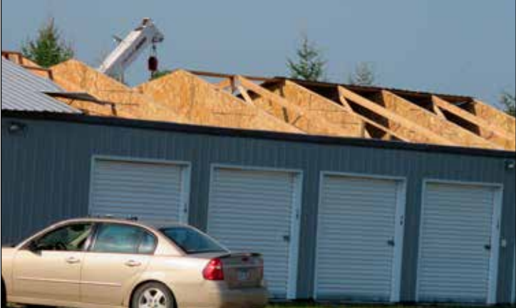
Roof off the storage unit across from the school in Clearbrook.
