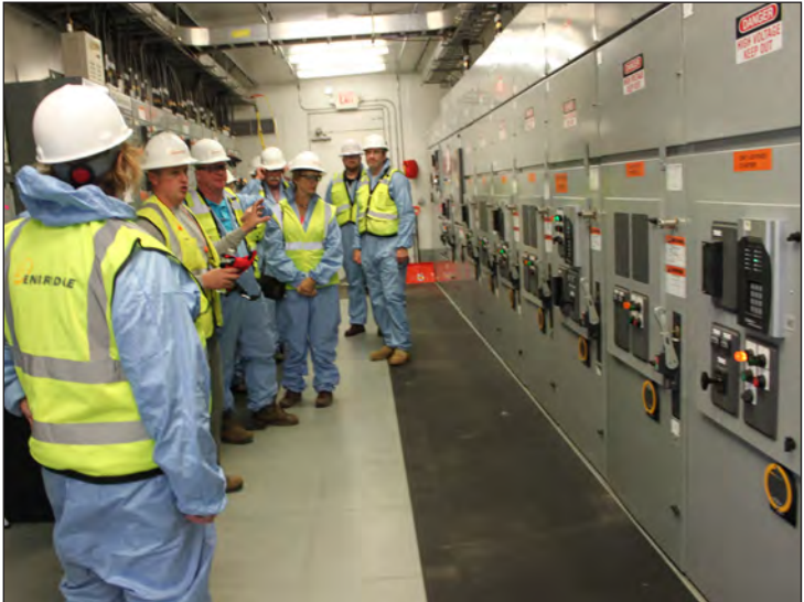
Inside the small building that houses the back up batteries and breaker boxes for Line 67 at the Enbridge pump station in Clearbrook.
