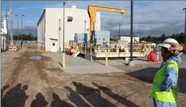
Building that houses Line 67 Project at Enbridge pump station near Clearbrook. As part of the Mainline Enhancement Program, Enbridge increased the average annual capacity of Line 67 in two phases, from 450,000 barrels per day (bpd) to its full design capacity of 800,000 bpd. The Line 67 Upgrade Project did not require new pipeline construction. Enbridge added pump station horsepower at the existing facilities.
