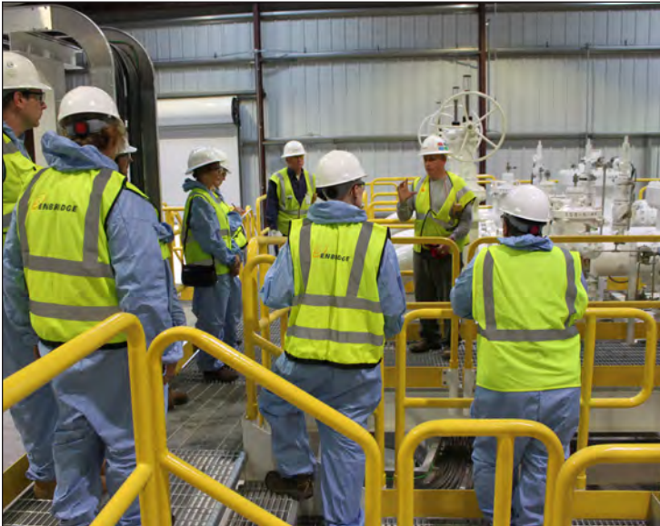
Ground valve controls are featured inside and outside of the Enbridge facility.
