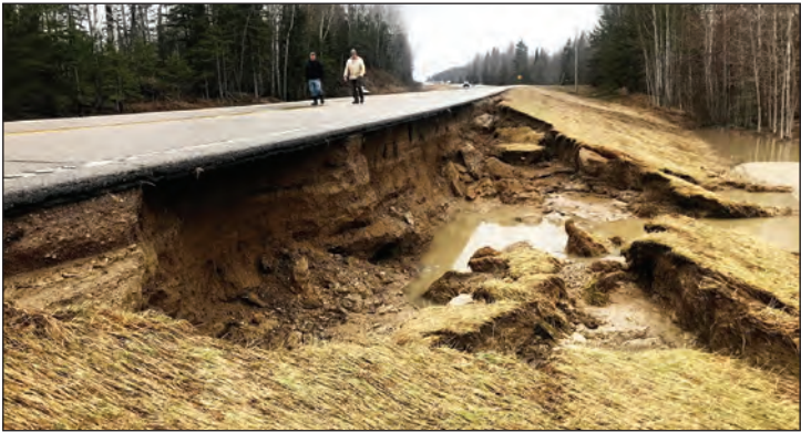
Be careful when coming to a wash out on the road. It may look fine but see the damage that is done under the road.
