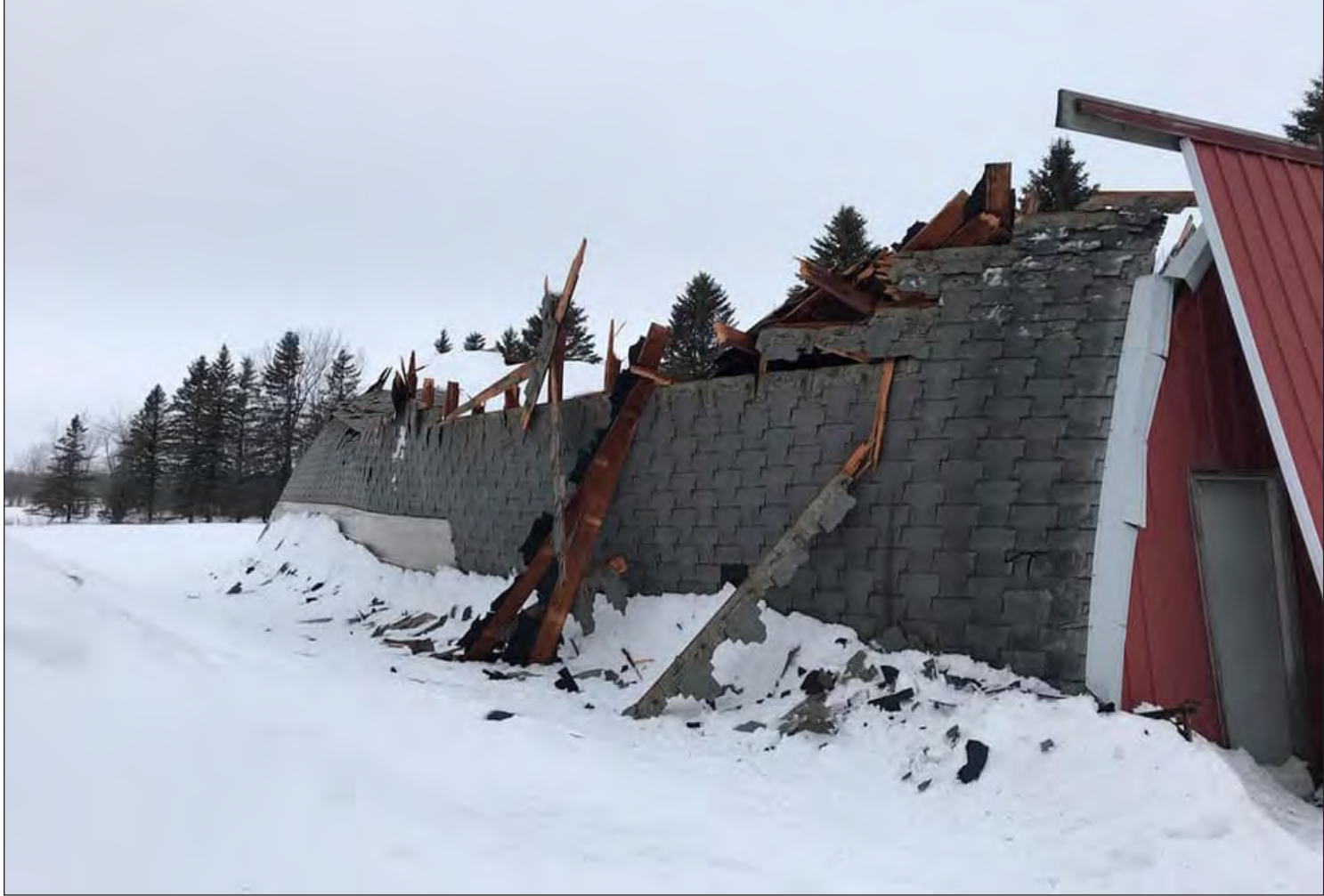
This 51-year-old 36'x77' quonset collapsed on the Ross Faldet farm near Clearbrook.
