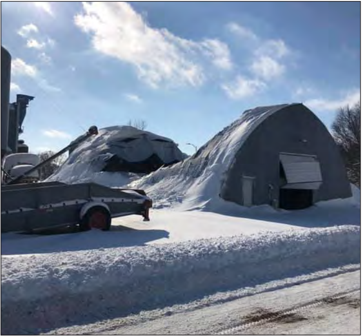
Fosston Tri-Coop lost a Quonset under the weight of the immense amounts of snow the area received in February and early March.
