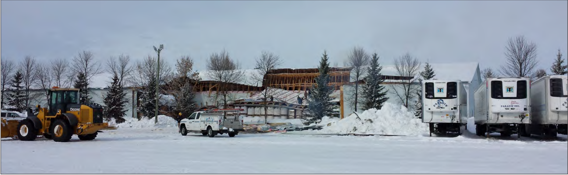
On Tuesday, February 12th in Brooks, the Paradis Warehouse had part of their roof collapse due to snow mostly likely. A large portion of the south side collapsed and clean up is underway.
